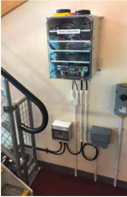
Virtual AIS unit installed at Shoreham RNLI station
