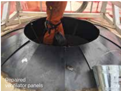
Rusting ventilator on lantern roof
