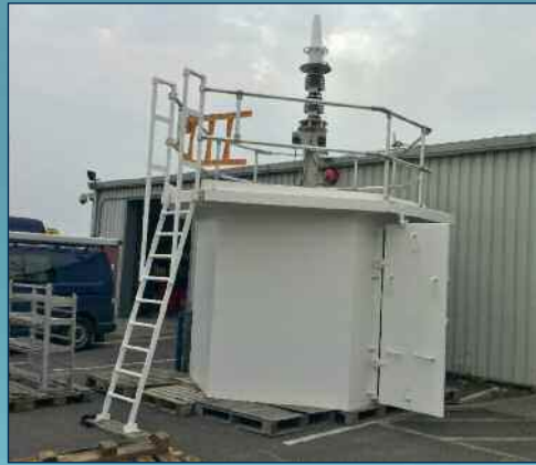
Above: Part of the electrical/ mechanical fit of new aids to navigation at Nab.
